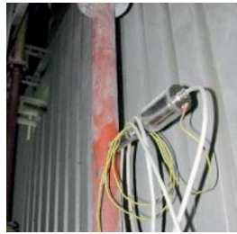
Adsorber / flue gas cleaning
